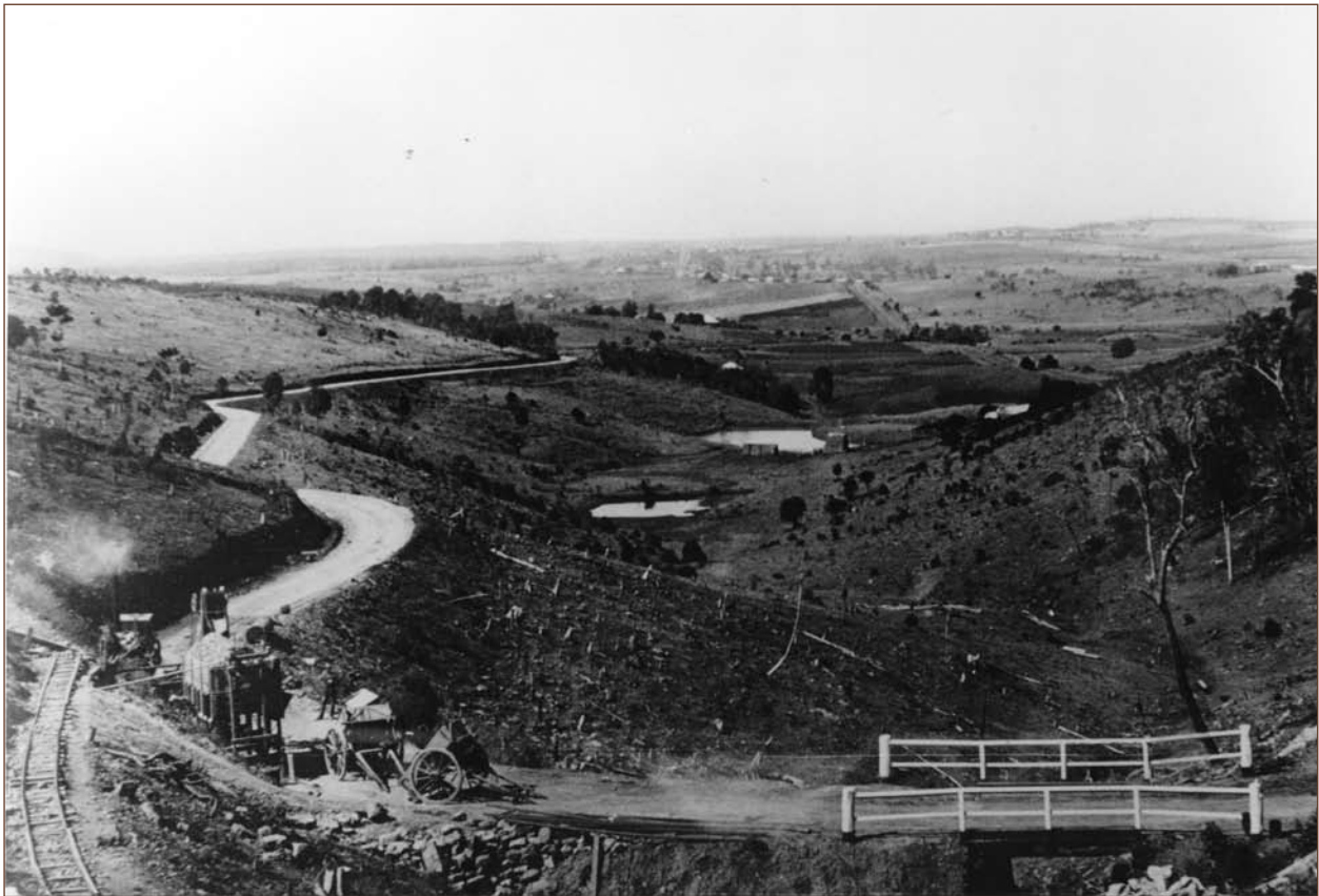
Building the “new” road over the range at Marburg. The route was altered again in the 1970s.
