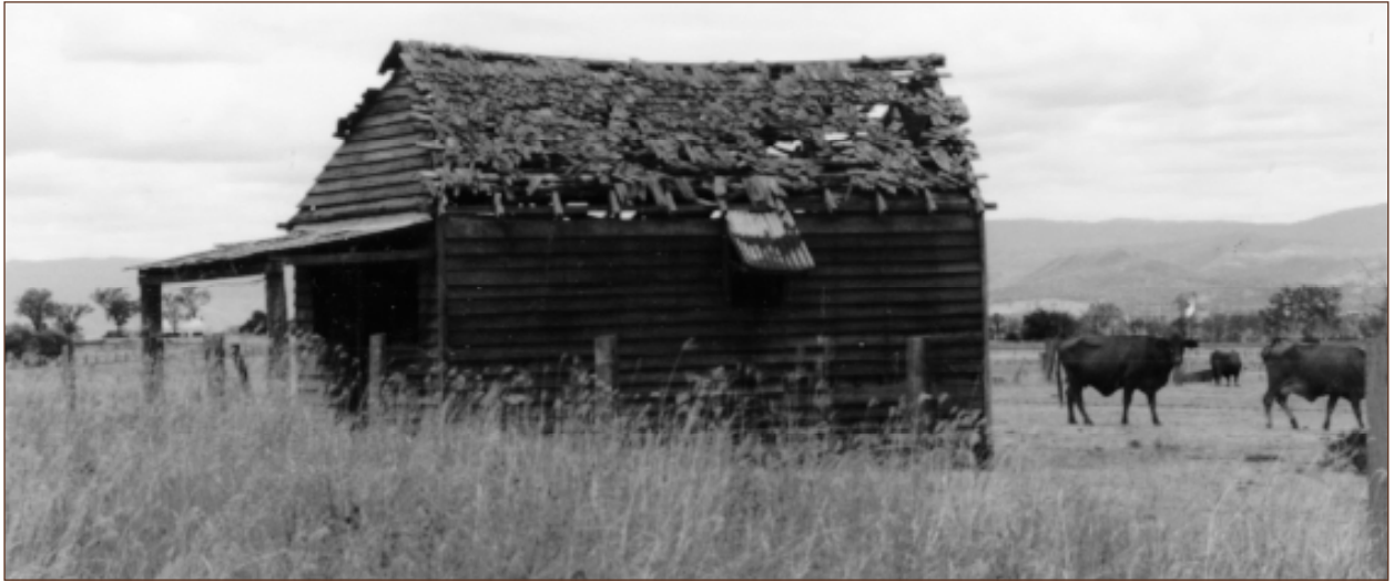
The old Butcher's Shop, Mt Walker West in the 1980s, before it collapsed
