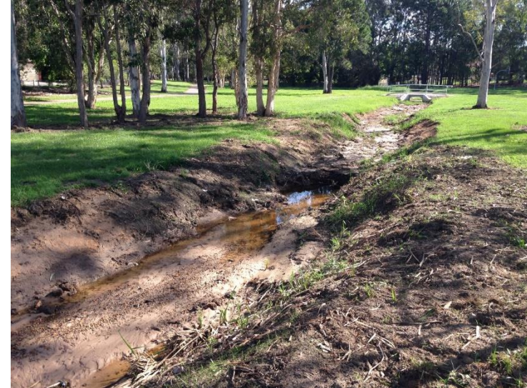
Erosion problems prevalent in Pollard Park pre-works contributing to elevated sediment and nutrient exports from the site
